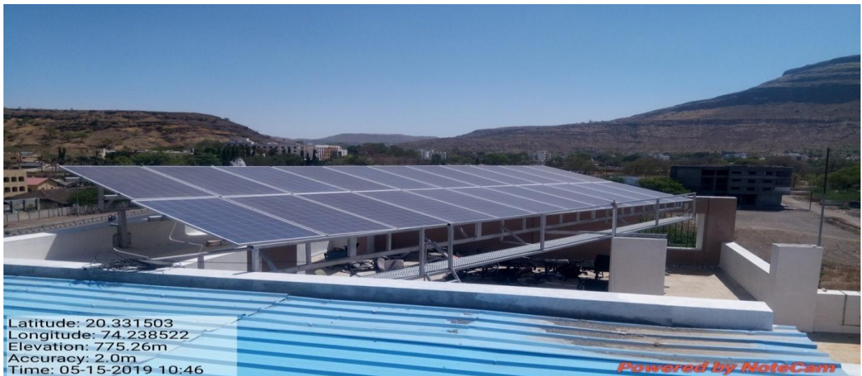
New Building Solar Panel
