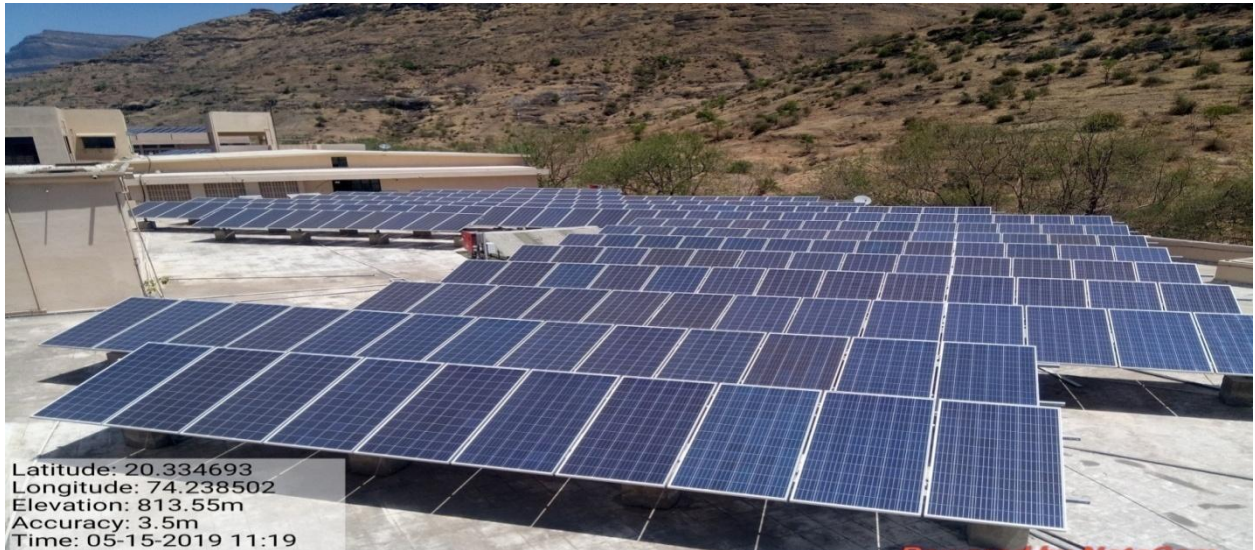
Chemistry Department Building Solar Panel
